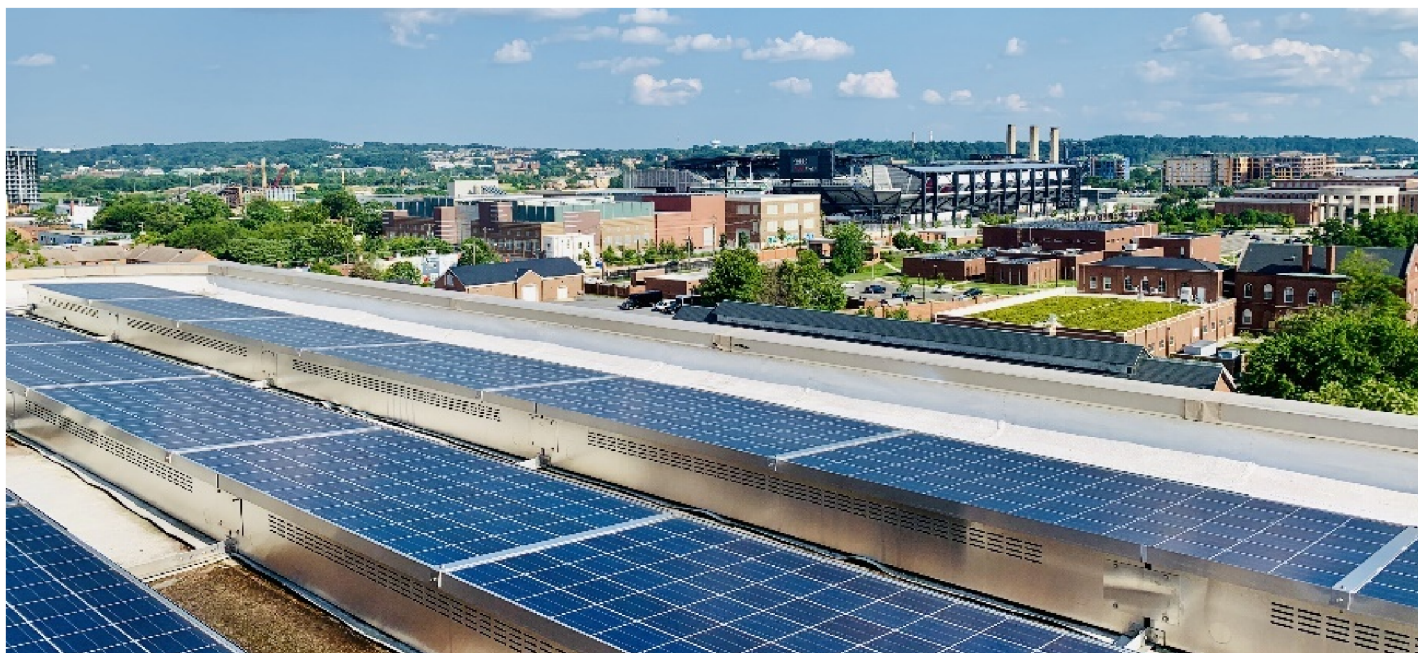
SOLAR ARRAY AT CHANNEL SQUARE APARTMENTS, WASHINGTON, D.C.
