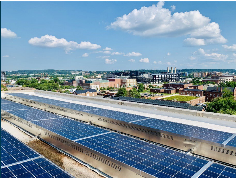
Solar Array at Channel Square Apartments, Washington, D.C.
